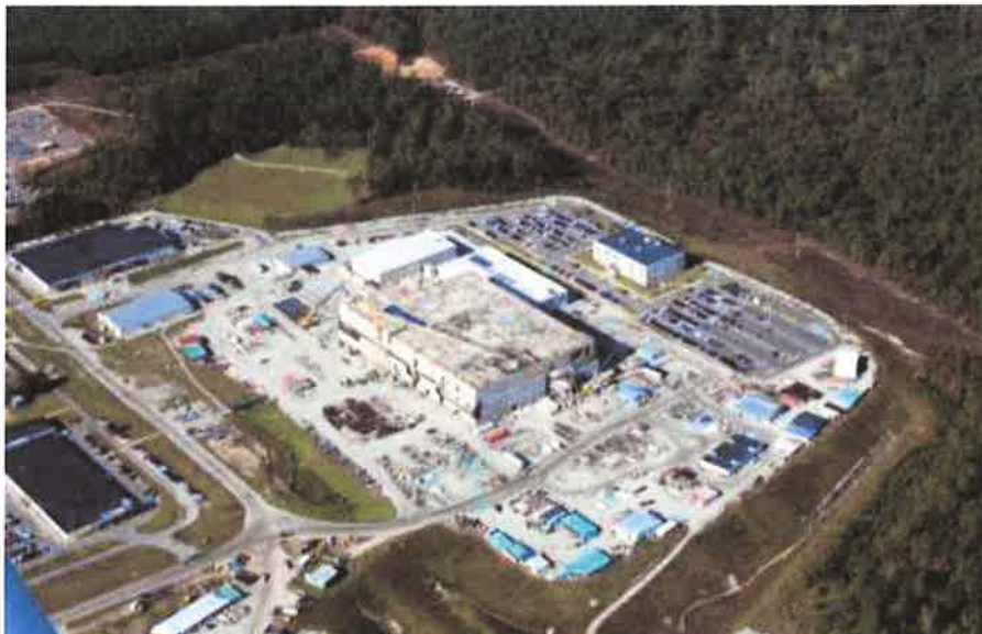
Photo: MOX plant under construction at SRS; note side of building facing left (south) – rusted rebar can be seen sticking out of top of unfinished gabion security wall, confirming that outside of MOX plant is not finished; October 25, 2014, by High Flyer, exclusive to Savannah River Site Watch
