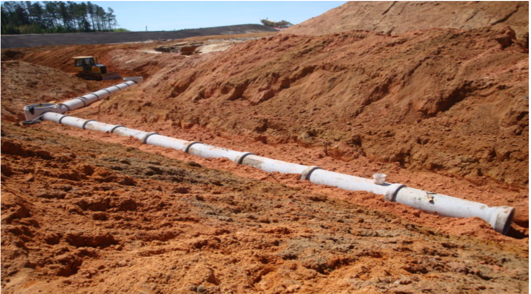
WSB Storm Sewer Piping
