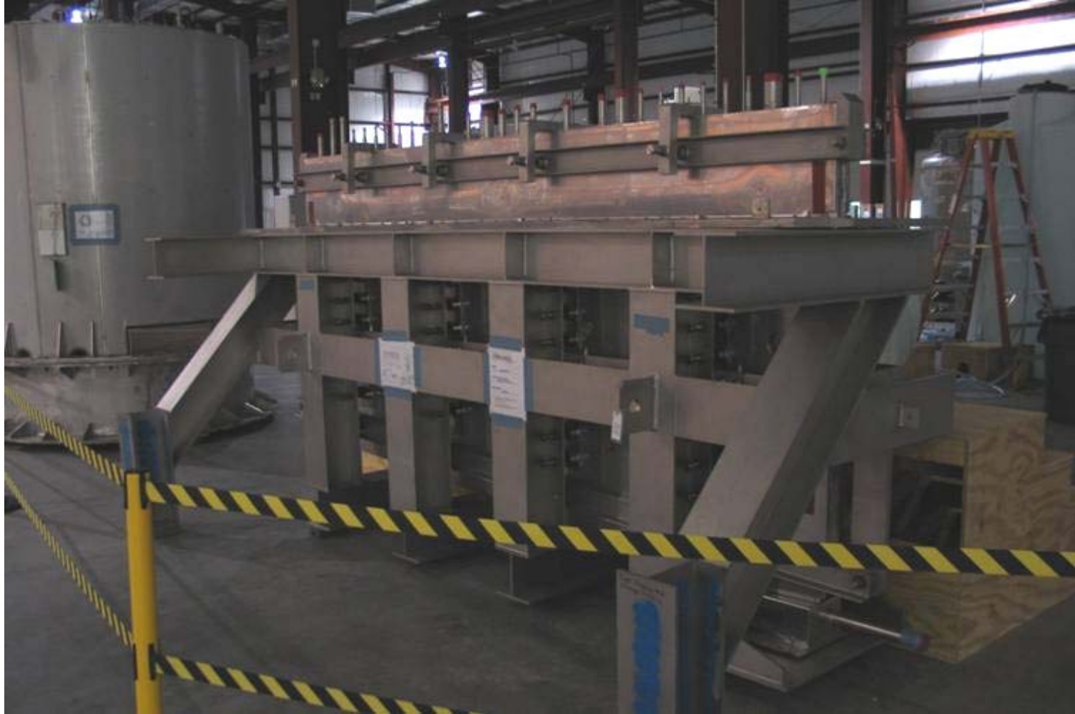
MFFF Process Tanks
