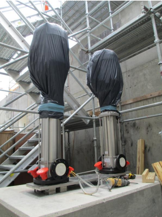
Aux Boiler Feed Pumps
