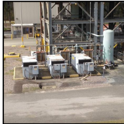
Saltstone Air Compressors
