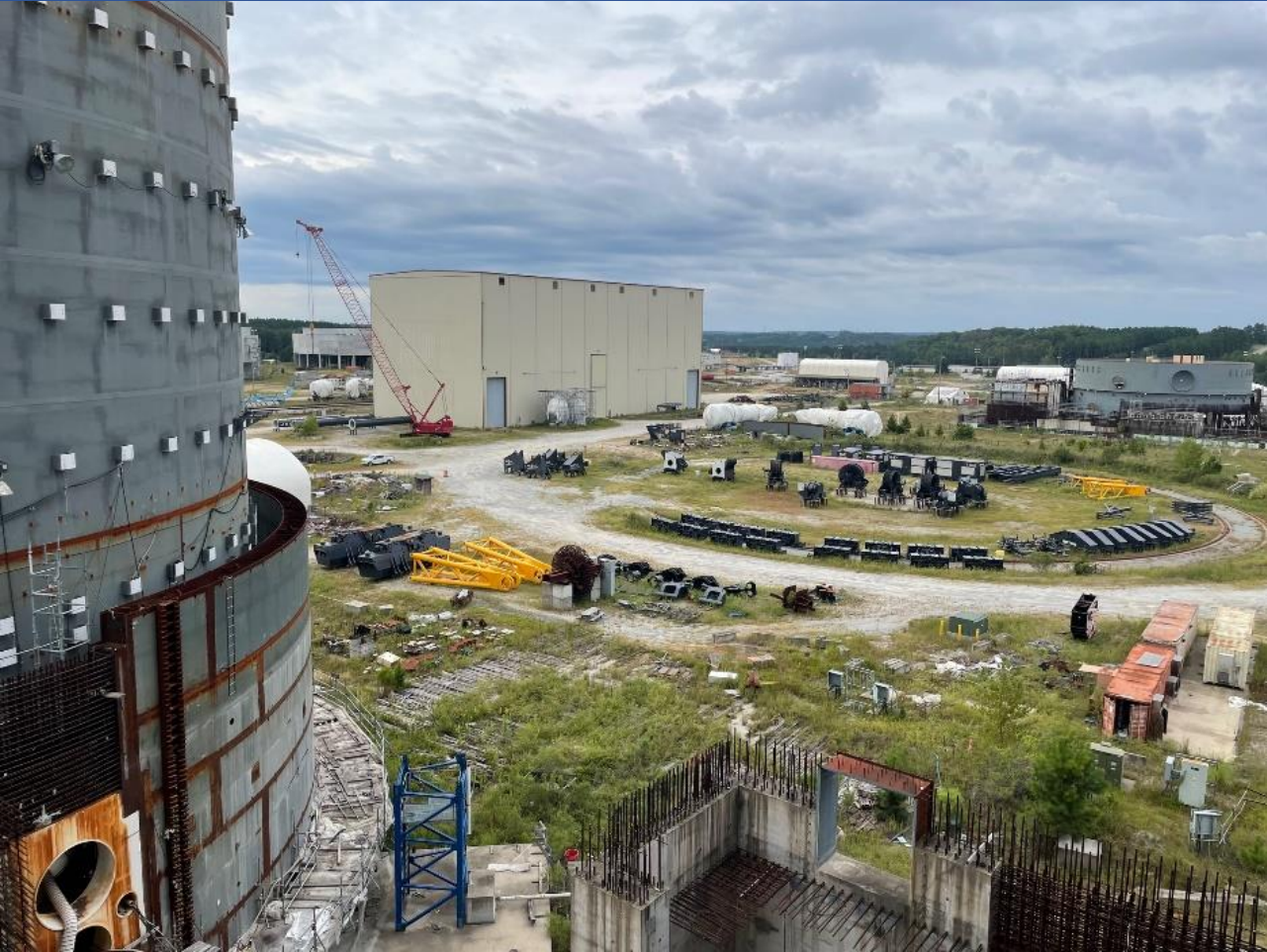
View from the Unit 2 Turbine Building towards the Modular Assembly Building and Unit 3 Containment Structure
