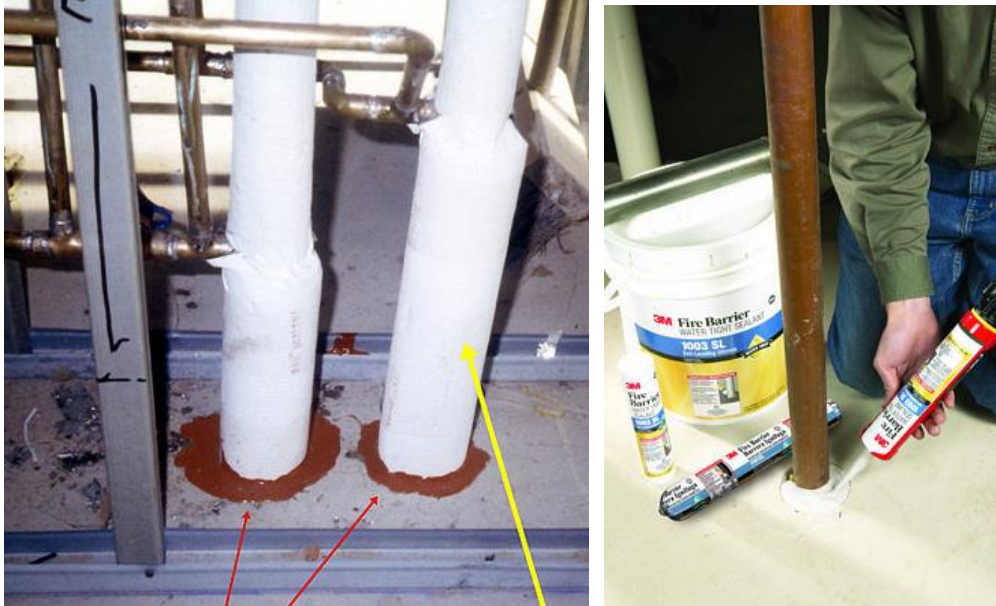
Silicone firestop with rock wool packing (red arrows) around mechanical pipes. Rock wool pre-molded insulation (yellow arrow) around pipes. Silicone sealant being applied (right photo).
