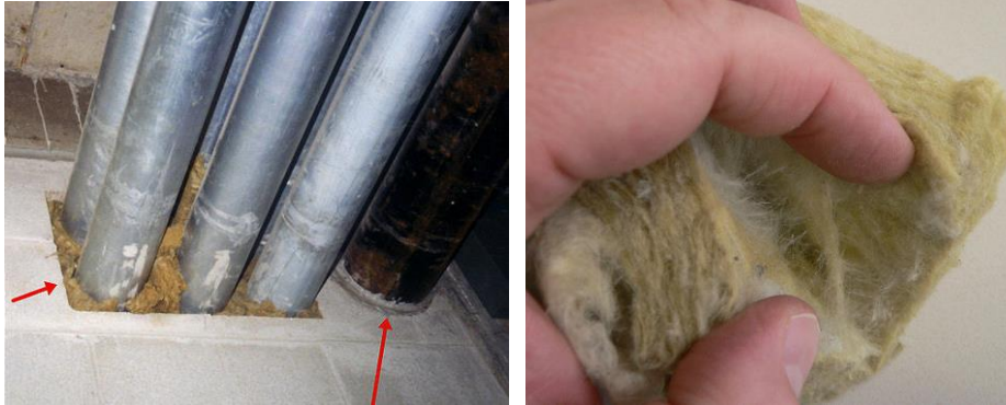
Rock wool (on left) is OK as packing but is missing overlying firestop. Firestop mortar is used around pipe (on right).
